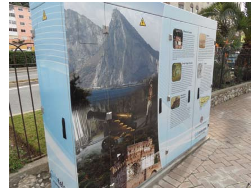
One of Gibtelecom's new beautified active street cabinets containing VDSL2 technology.
